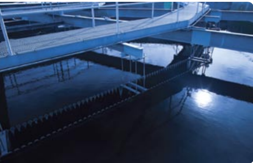
Sedimentation tank, Eastern Treatment Plant
