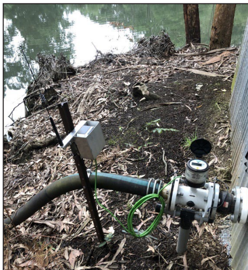
Figure 4: Siemens Mag8000 meter with data transmitter
