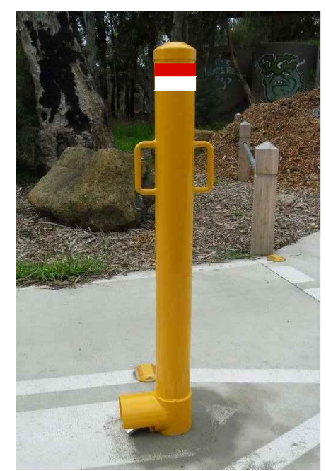
Photo 1 TYPICAL SINGLE LOCK BOLLARD – SIDE VIEW. BOLLARD INSTALLED IN SLEEVE CAST INTO CONCRETE SHARED PATHWAY.
