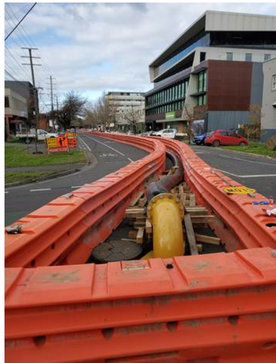
Sewerage bypass discharge into manhole 23
