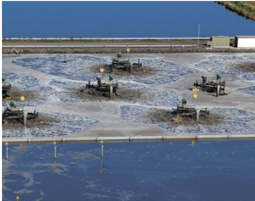
Western Treatment Plant aerators
