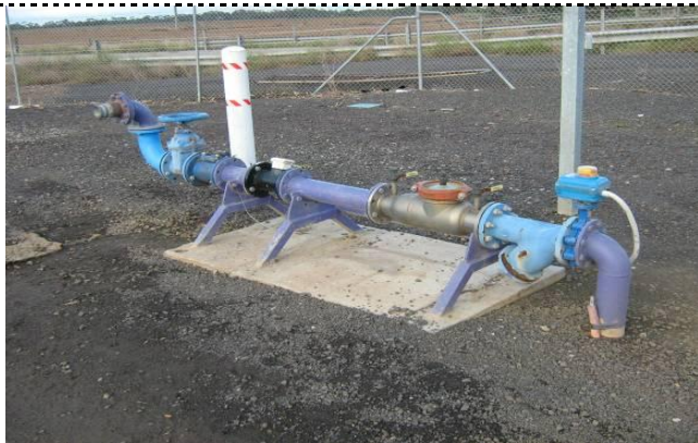
Recycled water standpipe
