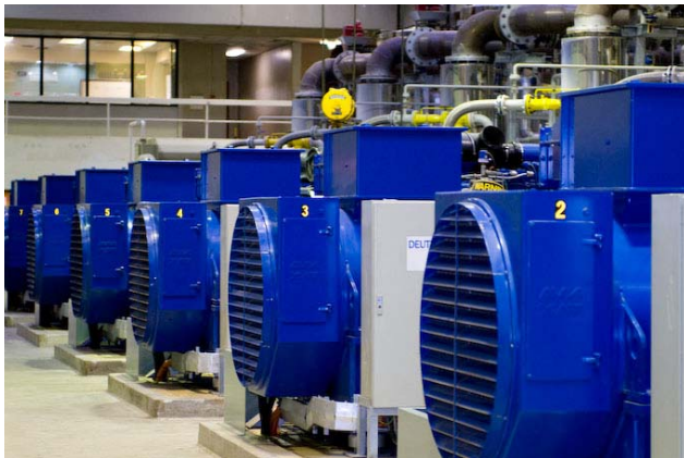
Power generators at the Plant can use biogas from the treatment processes. What will sewage treatment look like 50 years from now?
