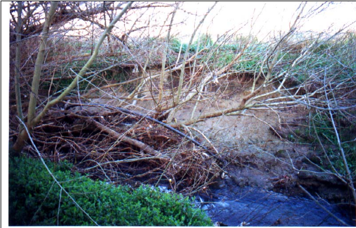
Figure 5: Willow obstruction and associated bank wash-out in Ferny Creek near Hancock Road
