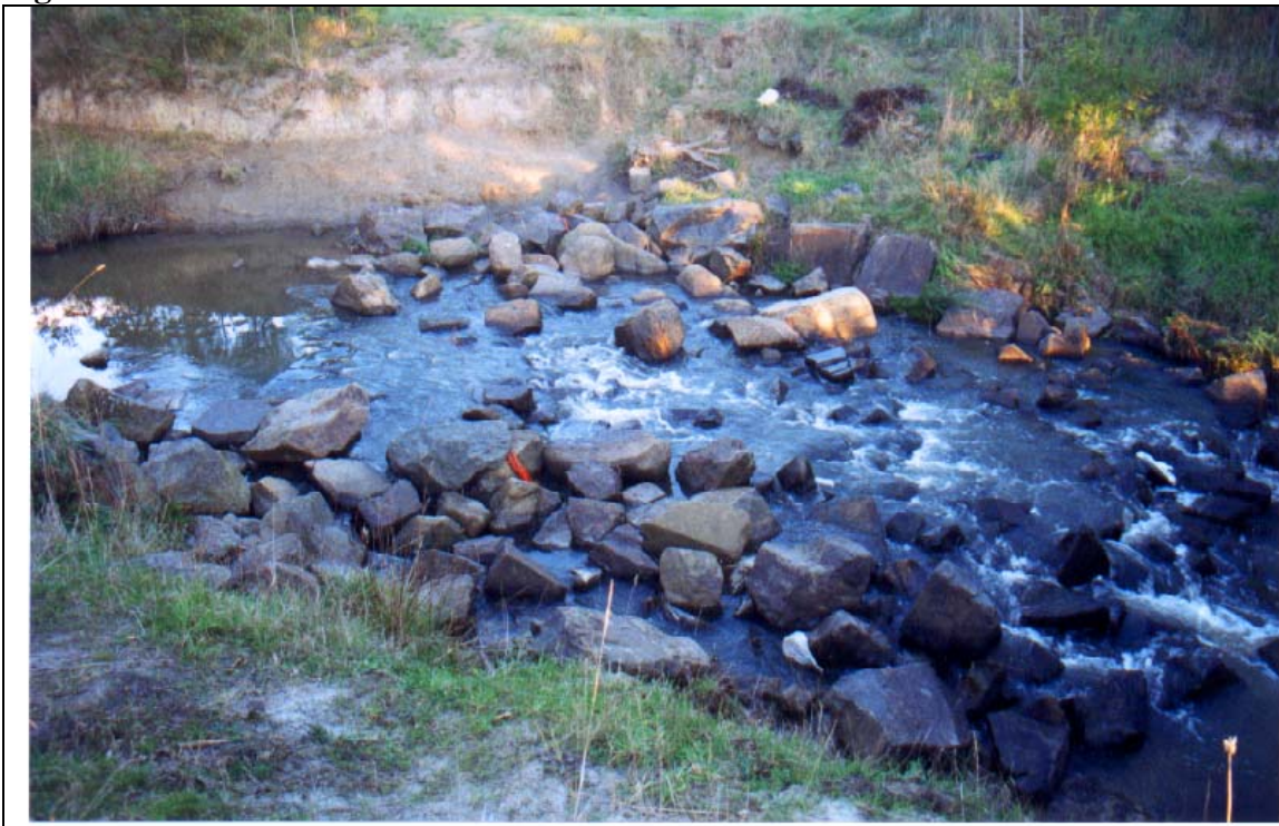
Figure 4: Bank erosion at a rock chute in Corhanwarrabul Creek
