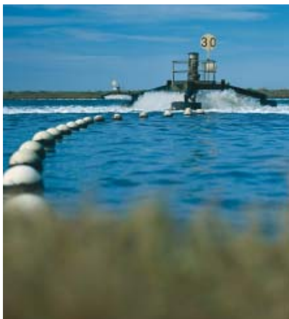
Aerators maintain oxygen levels in lagoons as part of the treatment process at the Western Treatment Plant.
