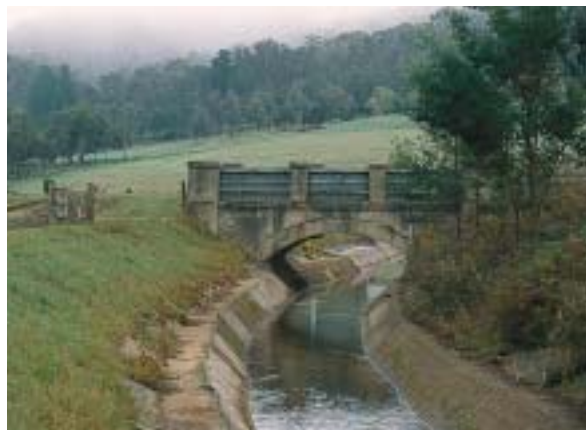
The Maroondah Aqueduct, which dates from the 1880s, is undergoing major work to reduce water leakage.
