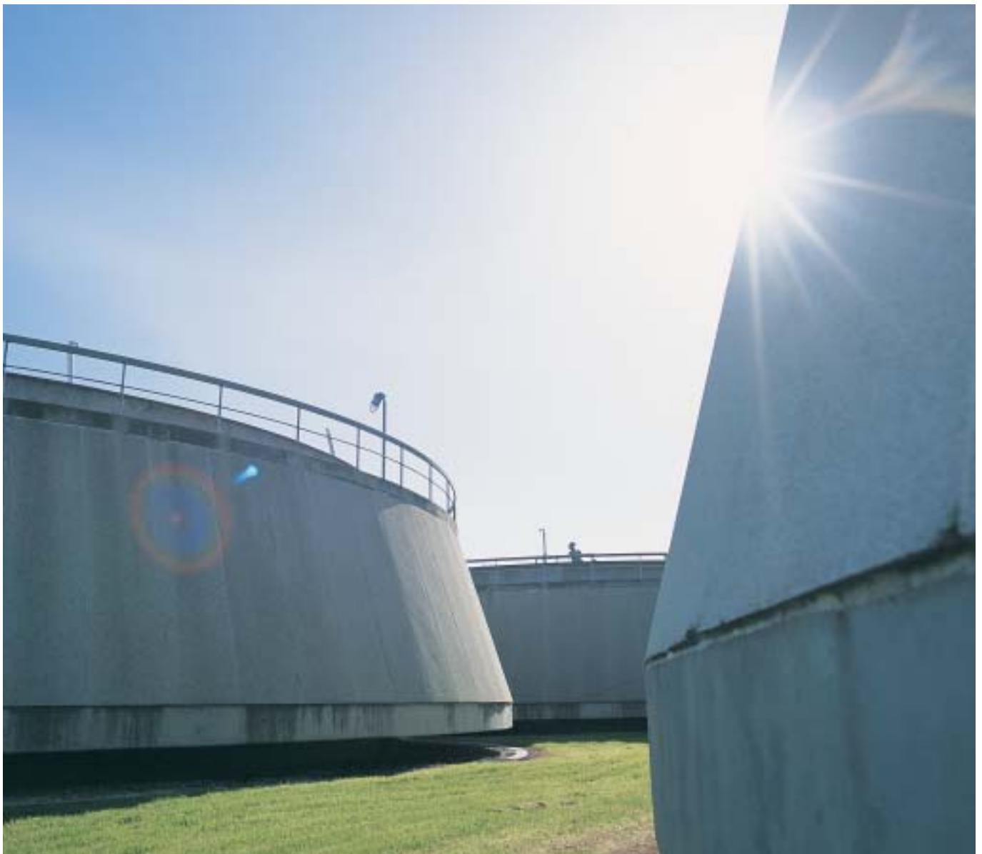
Modification of these digesters as part of the Eastern Green Energy project will reduce greenhouse gas emissions from the Eastern Treatment Plant by 24,500 tonnes per year.
