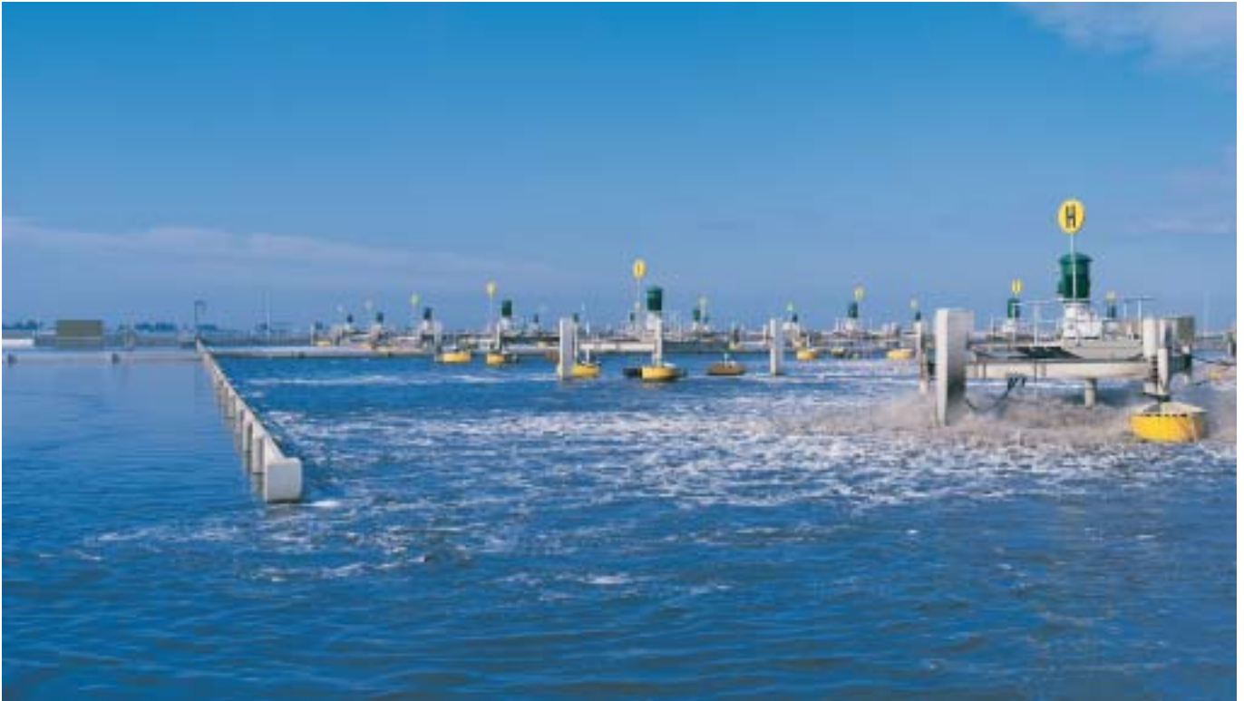
Lagoon 55 east at Western Treatment Plant is undergoing a major upgrade which, together with the planned second lagoon upgrade, is anticipated to reduce nitrogen to Port Phillip Bay by 500 tonnes per year.
