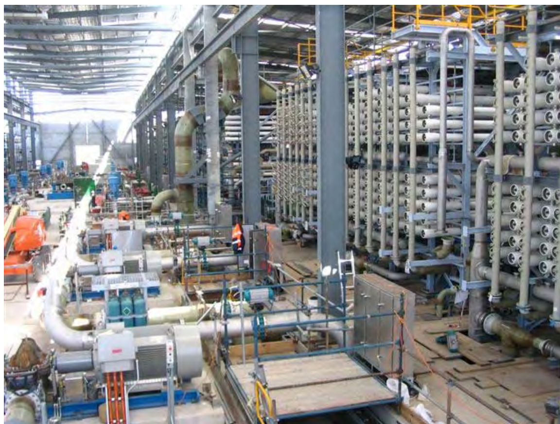
Figure 16 –Reverse osmosis racks inside a large seawater desalination plant (under construction)
