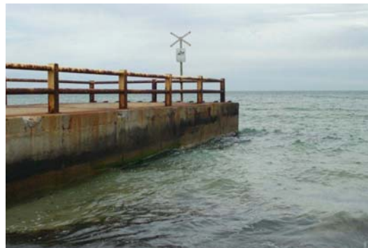
Figure 1 – The Riviera Street drain outlet is nearly 50 years old and in need of replacement
