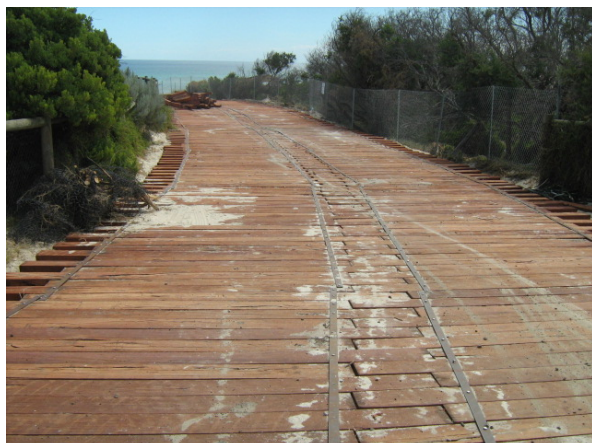
Red gum sleepers form a stable path for the safe movement of machinery to and from the beach
